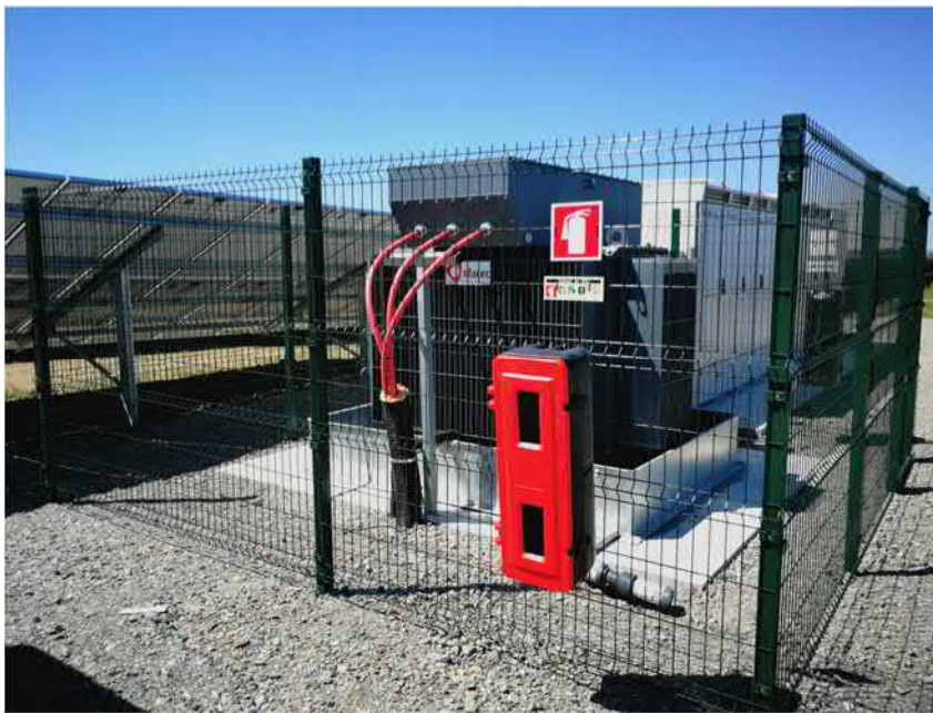
Photo 2-15: Typical transformer compound fencing
