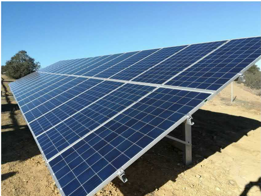
Photo 2-3: Solar panels with south facing configuration
